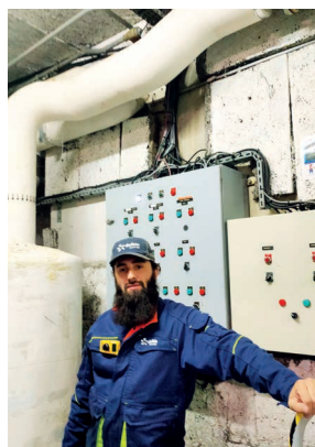
Steve Arrais – Heating technician / Dalkia Île-de-France region
